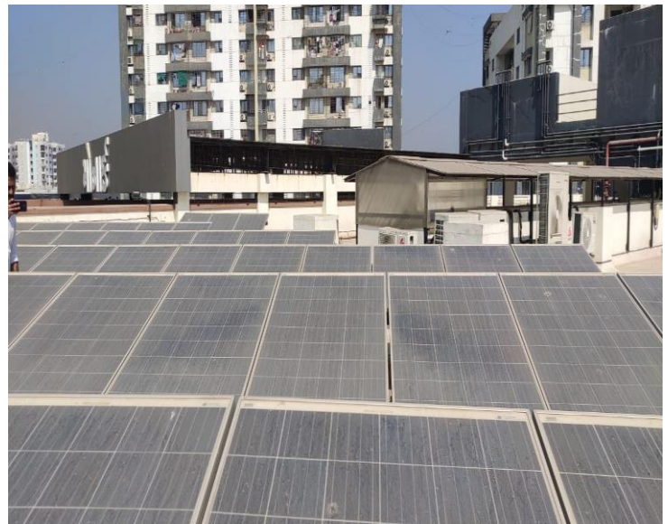
Solar panel system (66KW Panel)
